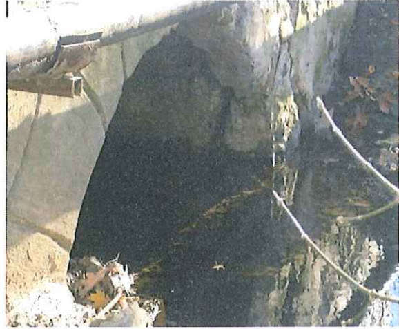
Failing Upstream Headwall in South Barrel
