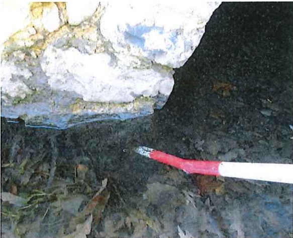
1'-0" Undermining at Outlet
