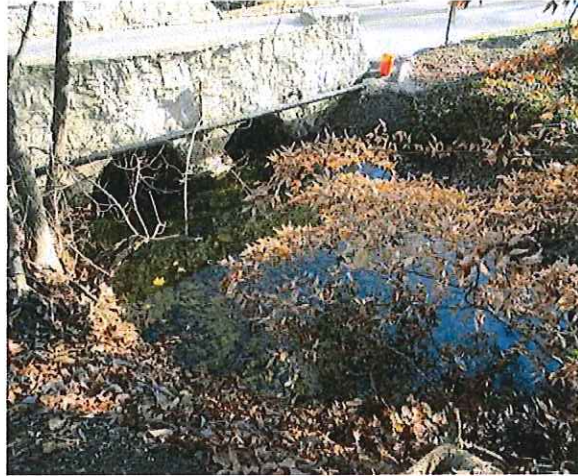
Large Scour Hole/Pond formed at Culvert Inlet
