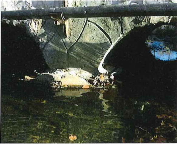
Undermining and Spall in Upstream Pier Footing
