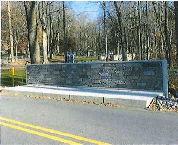
Sidewalk on a Newly Constructed Bridge along Chamounix Road over Branch of Gulph Creek
