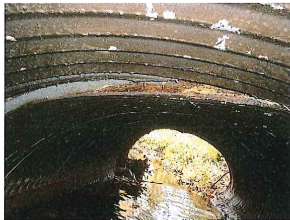
Upstream portion of East Pipe shows Excessive Deformation & Separation from Abutting Section
