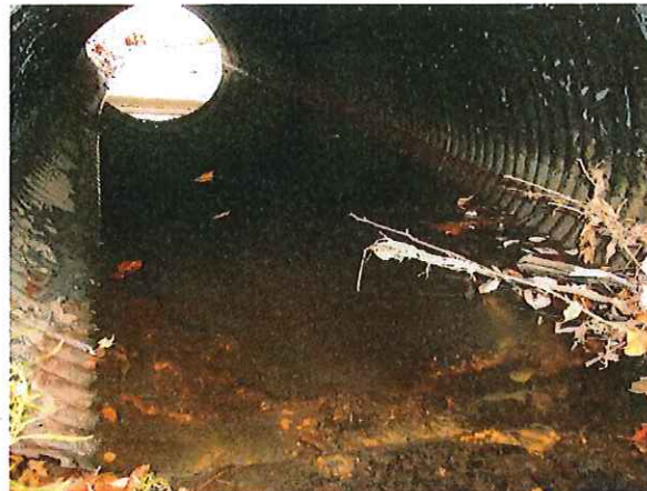
East Pipe with Apparent Heavy Rust
