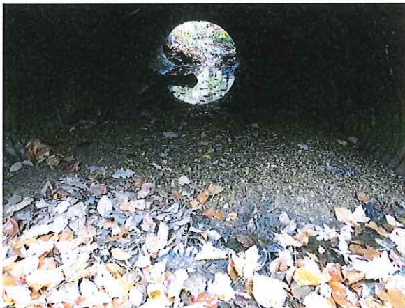
West Pipe with Heavy Silt Built-up
