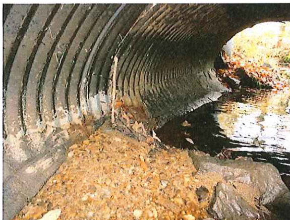
Misaligned/Distorted West Pipe Shows Loss of Fill Material
