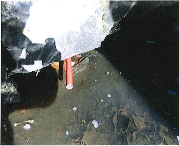
4' Undermining under North Abutment of Inlet Structure
