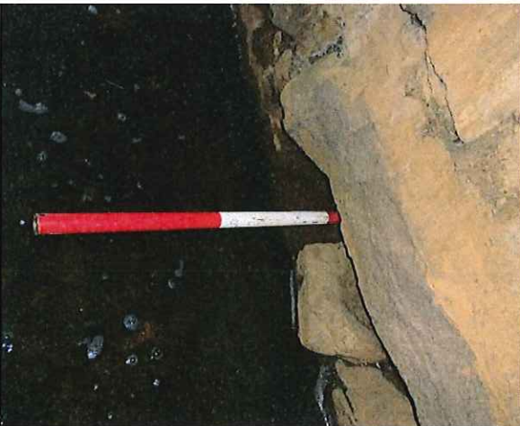
2' Deep Void in North Abutment
