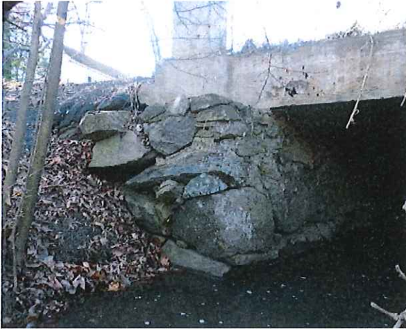
East End of South Stone Masonry Abutment, Note Large Stones with Missing Mortar Joints
