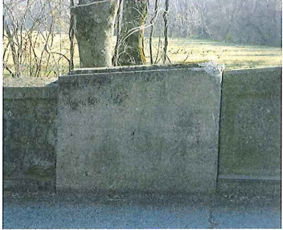
Spalls in Bridge Barrier
