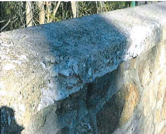
Spalls in Concrete Cap of Wingwall Barrier
