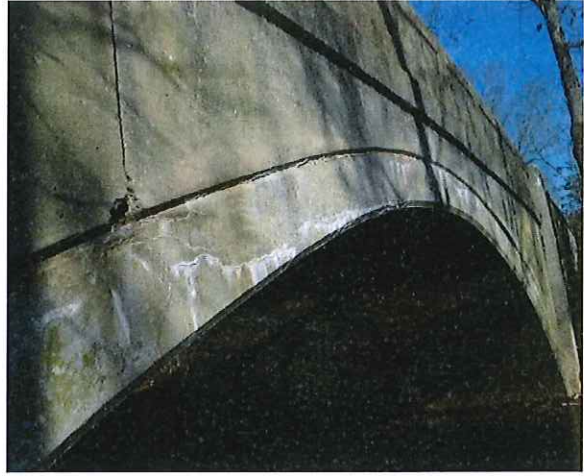
Small Spall in South Spandrel Wall and Fine Map Cracks with Efflorescence in South Fascia of Arch Barrel
