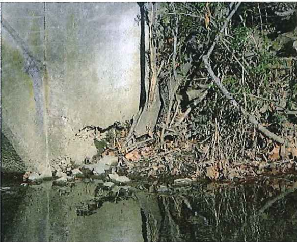
Large Spall at Bottom of Southeast Wingwall
