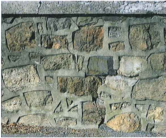
Cracks in Wingwall Barrier
