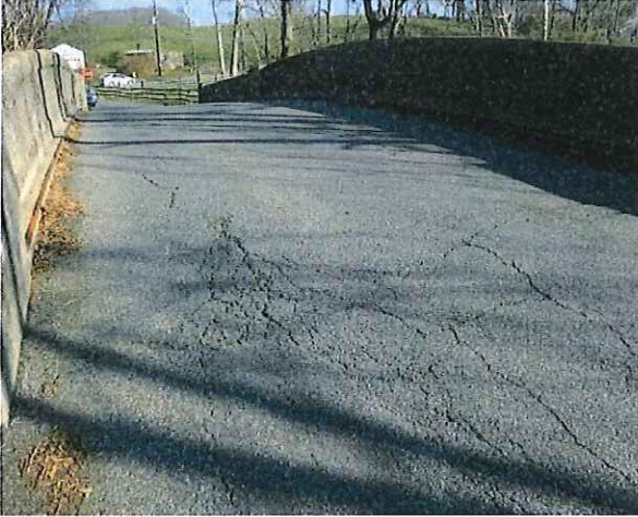
View of Pavement – Cracks throughout
