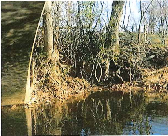
Bank Erosion with Exposed Tree Roots in Bank of Southeast Corner of the Bridge
