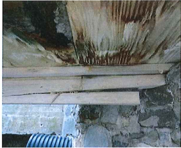
Large Hole in Deck and Horizontal Split in Stem of T-Beam
