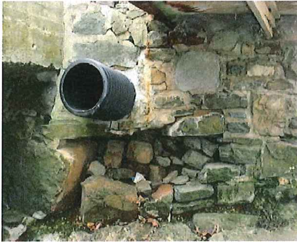
Missing Stones and Undermining in Wing D
