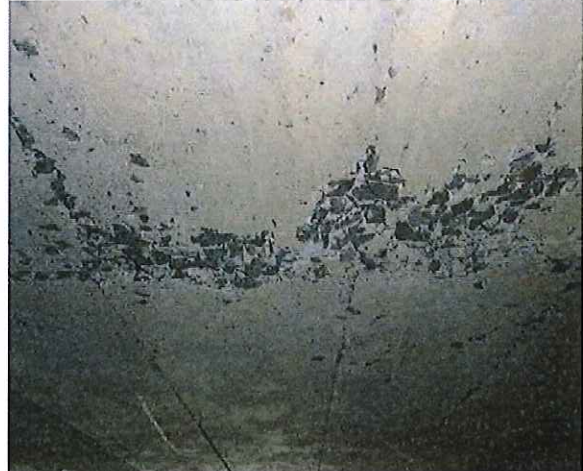
Honeycombing and Exposed Aggregate
