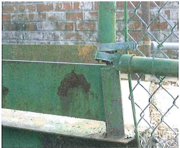
Broken Railing Post in N. Railing of North Pedestrian Bridge
