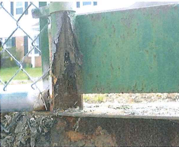
Section Loss in N. Railing Post of North Pedestrian Bridge
