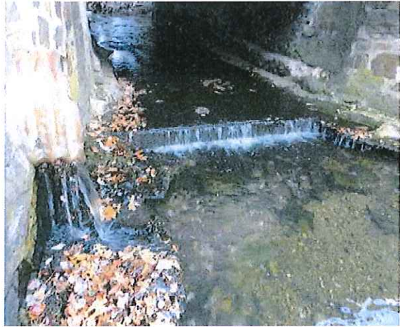
Large Scour Hole at end of Culvert
