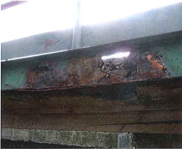
100% Loss in Web of North Stringer
