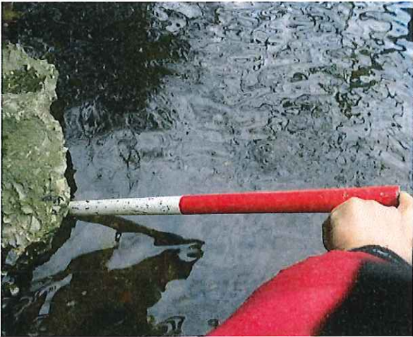
2' Undermining under Wing B Apron
