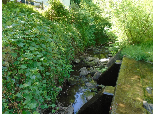
General View of Gabion Wall (left) prior to failure (conc. abutment sewer encasement in right foreground)
