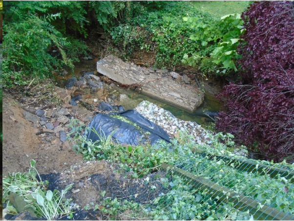
Failed stone wall, west bank w/exposed sewer
