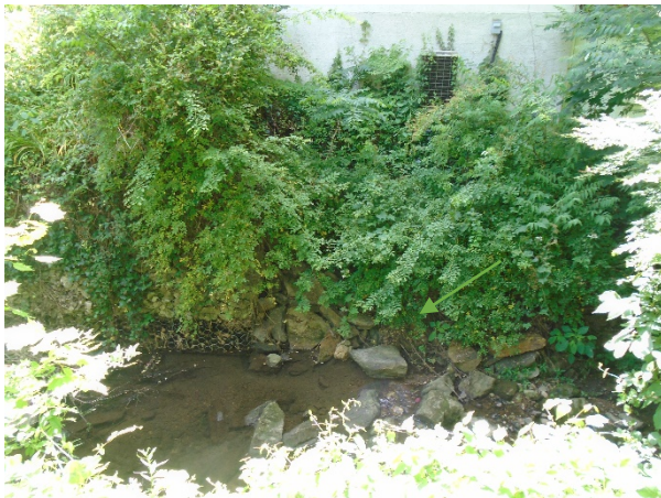
End of Gabion wall prior to failure
