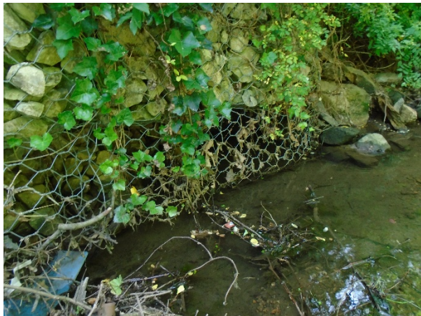
Undermining of gabion wall prior to failure
