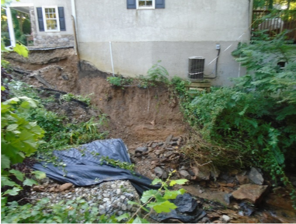
End of Gabion wall after failure, exposed wall
