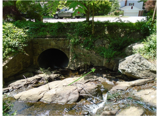
Upstream wingwalls - undermined
