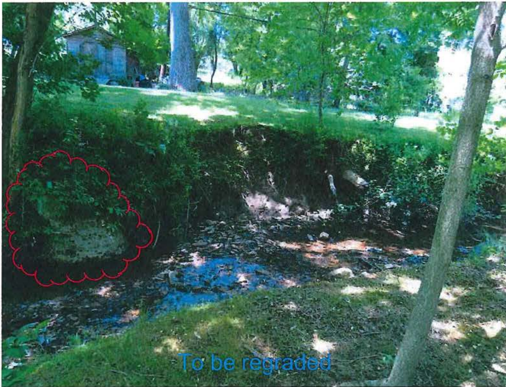
Photo 1. Manhole within stream channel and eroded sewer line ROW.
