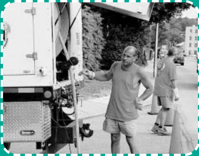
Members of a public works crew install and test a sanitary sewer line.
