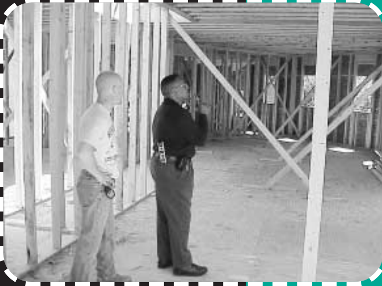
Codes Official Larry Taltoan (right), one of the Township's inspectors, conducts one of the required inspections for a new home. New construction in Radnor Township is subject to five inspections: footing, foundation, backfill, framing, and final.
