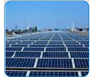
On-roof PV plants
